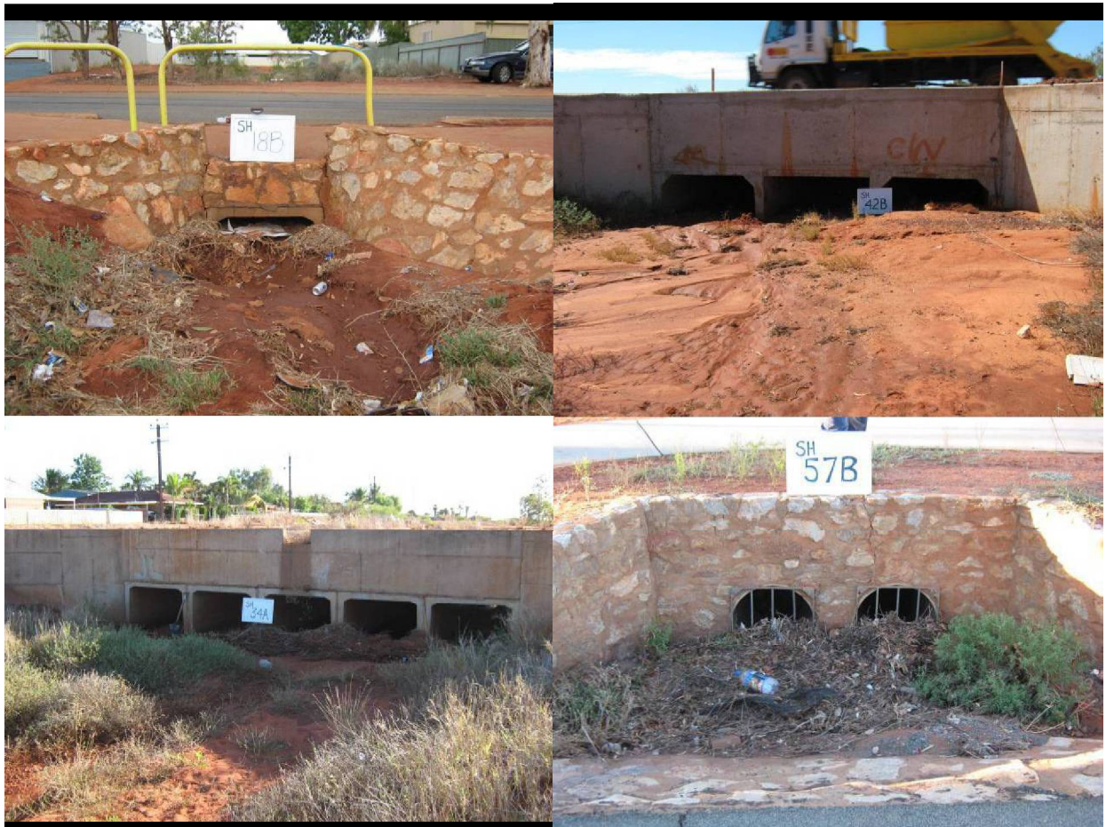
Plate 1 – Culvert Obstructions (SH18, SH42, SH34 and SH57)
