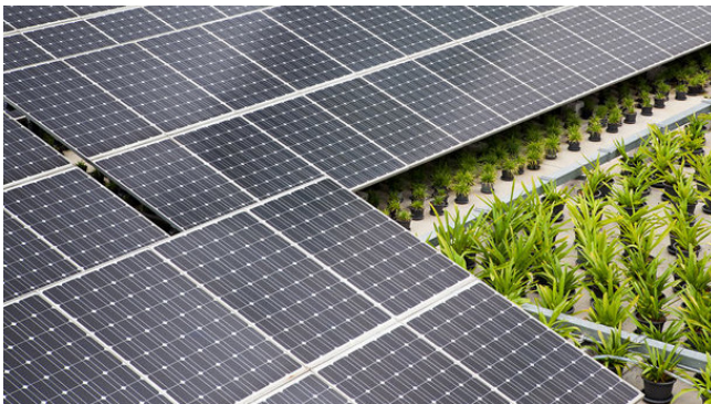
Roof mounted photovoltaic cells.
