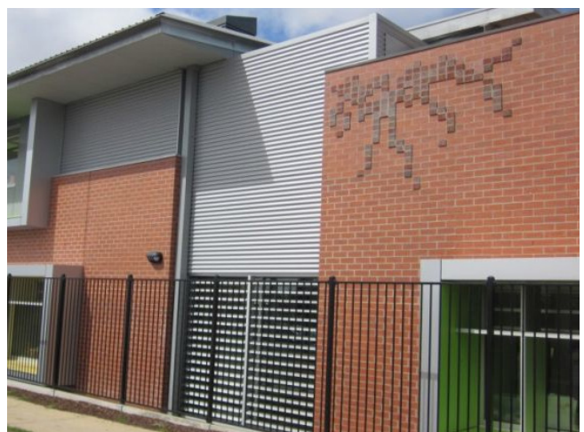
Examples of service enclosures and screening treatments designed as an integral part of the overall development.
