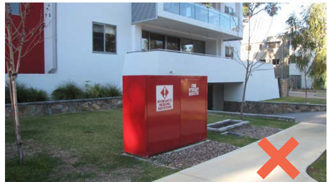
An example of the fire hydrant booster located as an afterthought.
