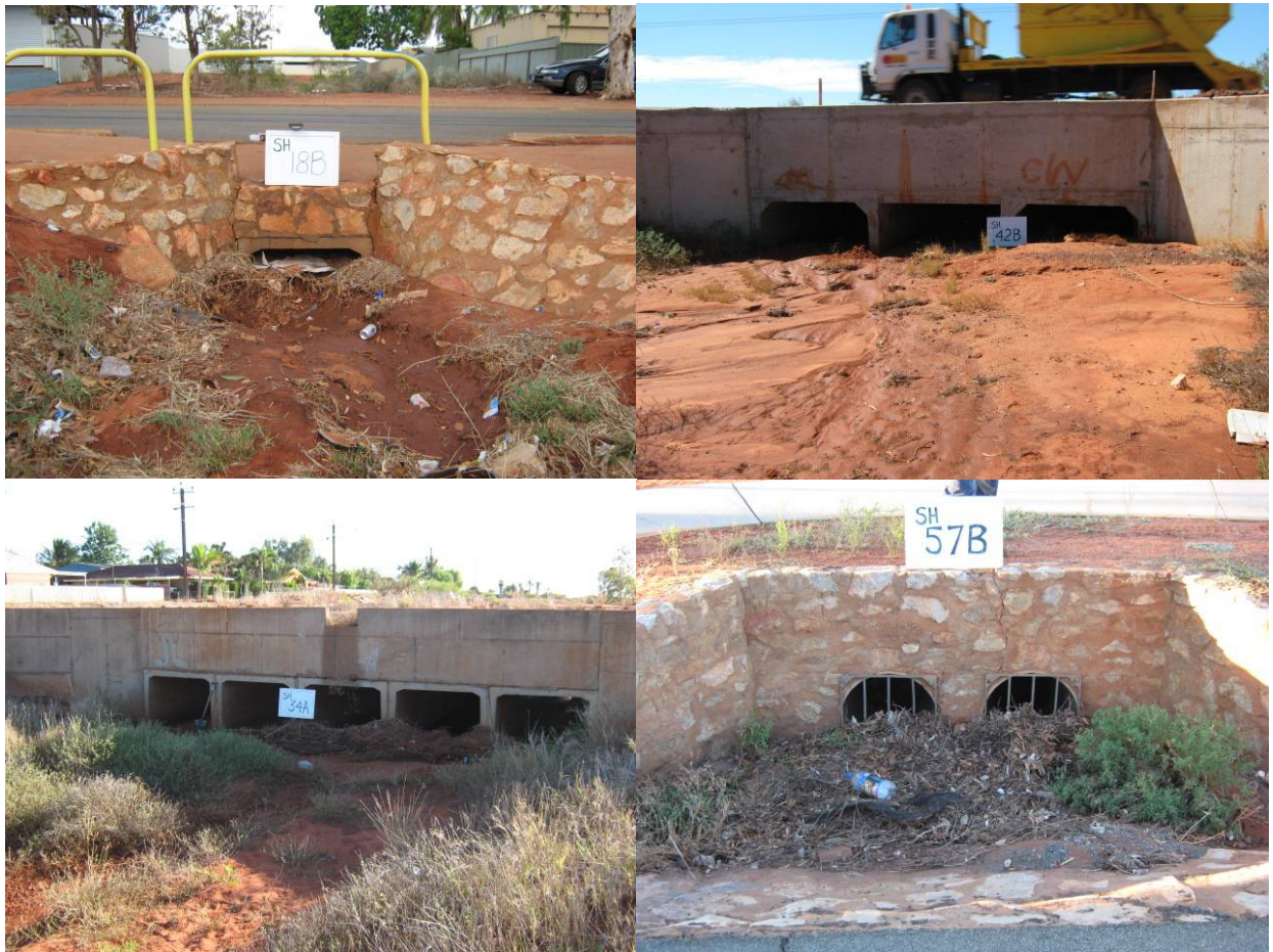
Plate 1 – Culvert Obstructions (SH18, SH42, SH34 and SH57)
