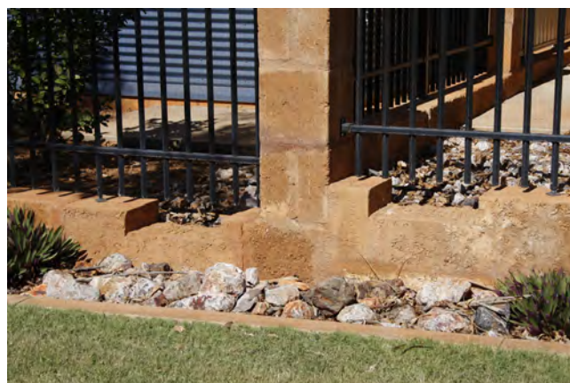
An example of controlling and minimising overflow and flooding through simple detailing, in this instance it allows for overflow from a small courtyard.
