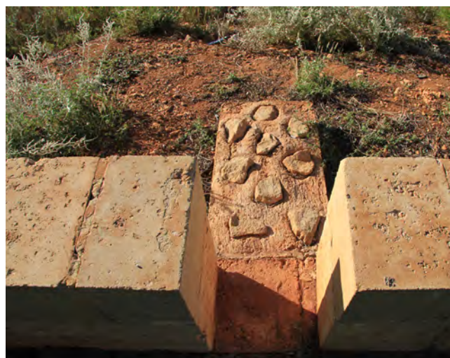
An existing good example of controlling overflow through simple wall detailing in a public park in Port Hedland.
