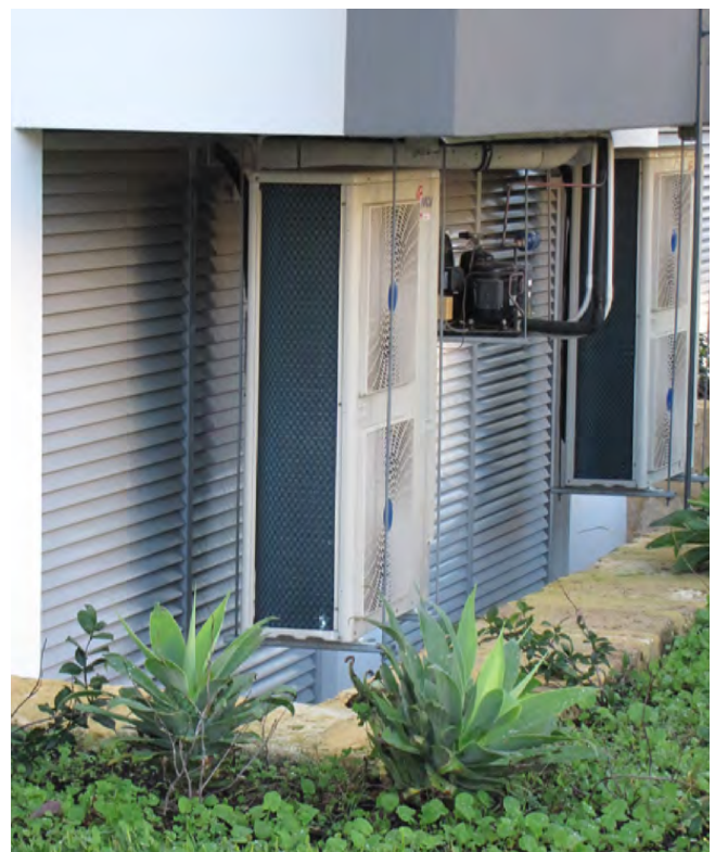
Air conditioning units located discretely and away from outdoor dining areas.
