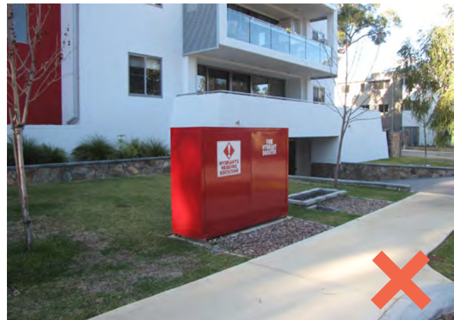
An example of the fire hydrant booster with a poorly designed outcome.
