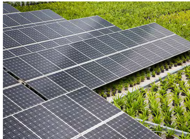
Roof mounted photovoltaic cells.
