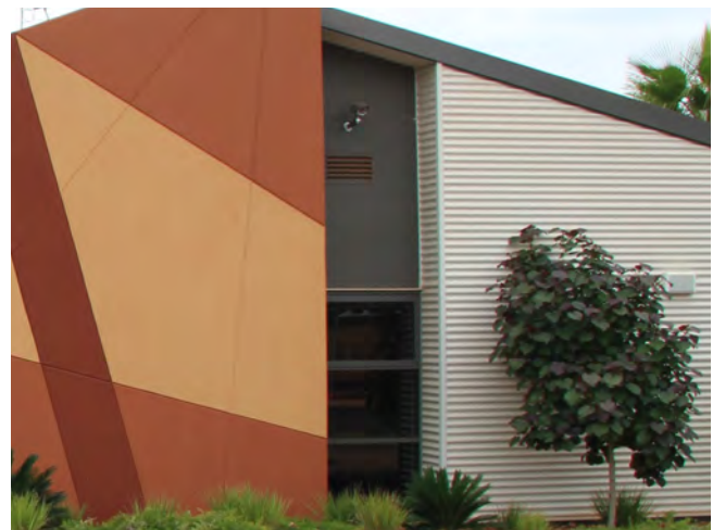
Utilising building design by recessing windows is an alternative option for providing shading to glazing.
