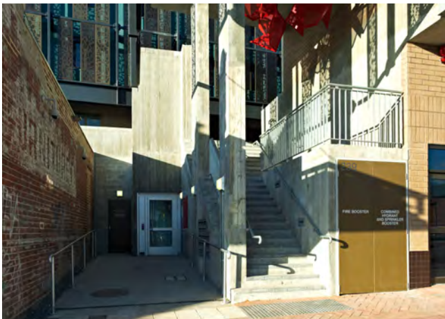
An example of fire hydrant booster well integrated into the building design.
