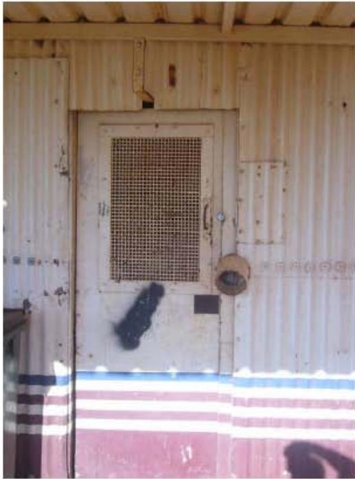
Photograph 9 East Elevation showing entry door McGregor Street Shed, Port Hedland Carrick + Wills Architects February 2010
