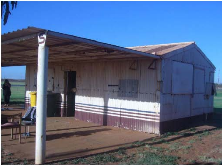
Photograph 1 North & East Elevation McGregor Street Shed, Port Hedland Carrick + Wills Architects February 2010
