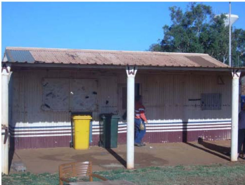
Photograph 8 East Elevation showing flat roof verandah McGregor Street Shed, Port Hedland Carrick + Wills Architects February 2010
