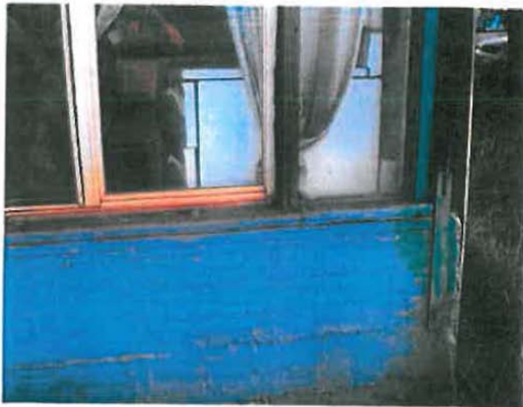
Front of southeast corner (kitchen) showing off form concrete and steel bracing detail.
