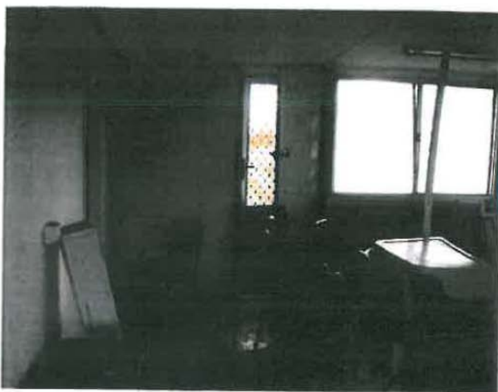
Interior: View looking into the north extension where the wall has been removed, showing the metal angle connection between ceiling and remnant wall.
