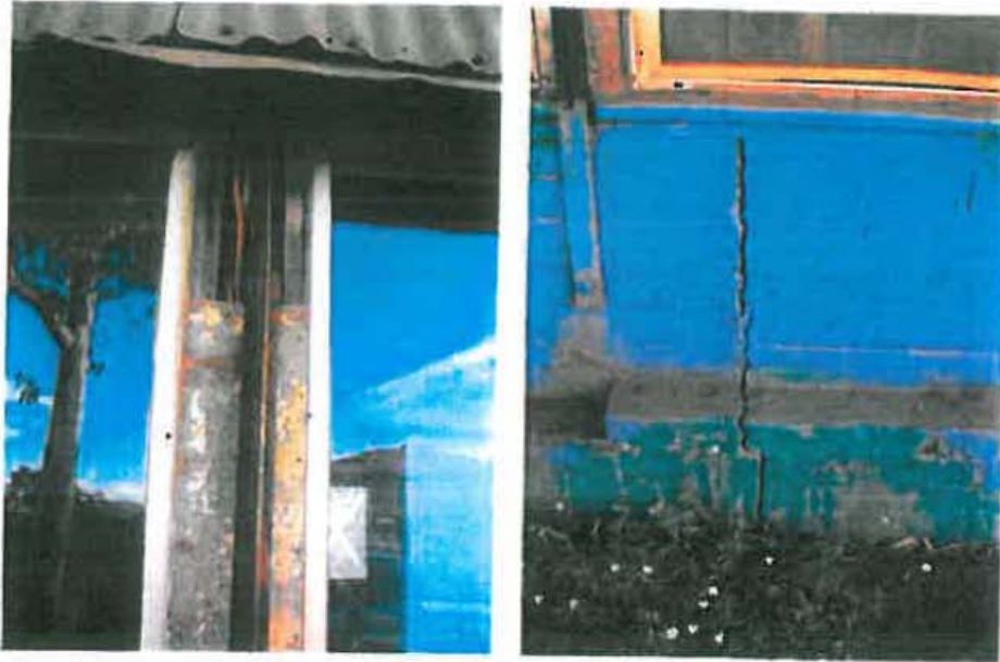
Front detail showing adhoc nature of the Interventions; structural cracking.
