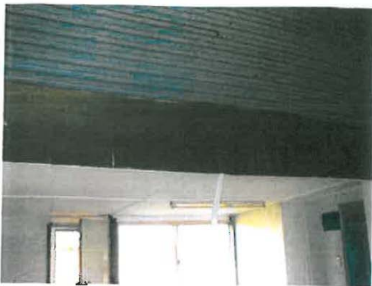
Interior: View looking into the north extension where the wall has been removed, showing ceiling levels and linings.
